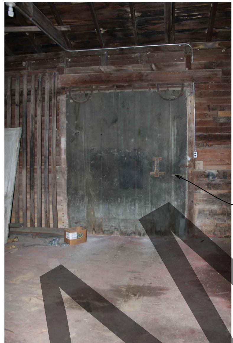
9 DEMO / EXISTING PHOTO AD-301 Not to Scale REMOVE ALL BARN DOORS AND HARDWARE
