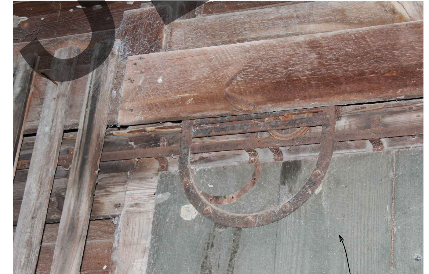
8 DEMO / EXISTING PHOTO AD-301 Not to Scale REMOVE ALL BARN DOORS AND HARDWARE
